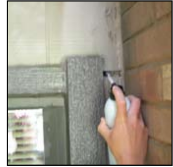
Inject voids containing carpenter ants or other void dwelling ants.
